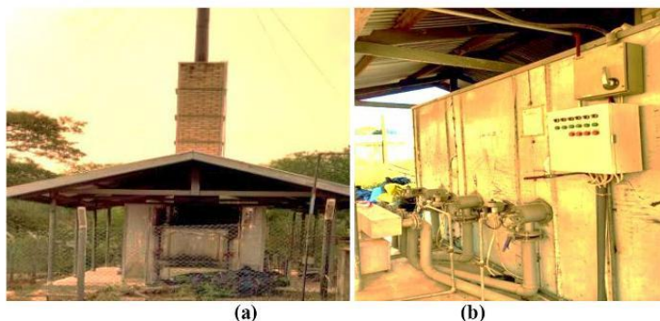
Fig. 1 Six-cylinder gas incinerators: (a) front view and (b) cylinder regulators
